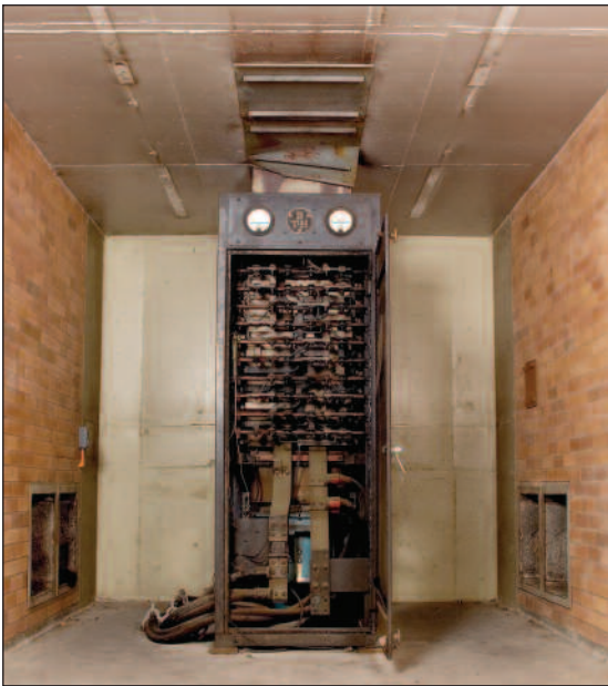
QR's original Load Bank at Redbank, Queensland
