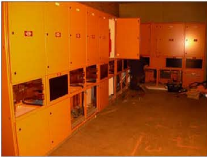
L-Shaped Modular Switchboard
