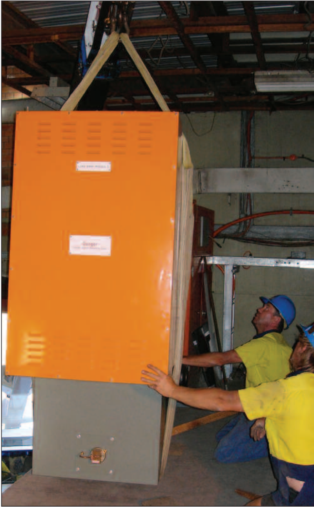
Installing the Load Bank module
