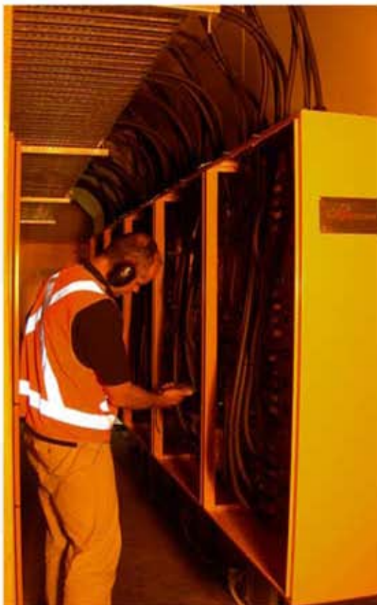
Commissioning of Load Bank
