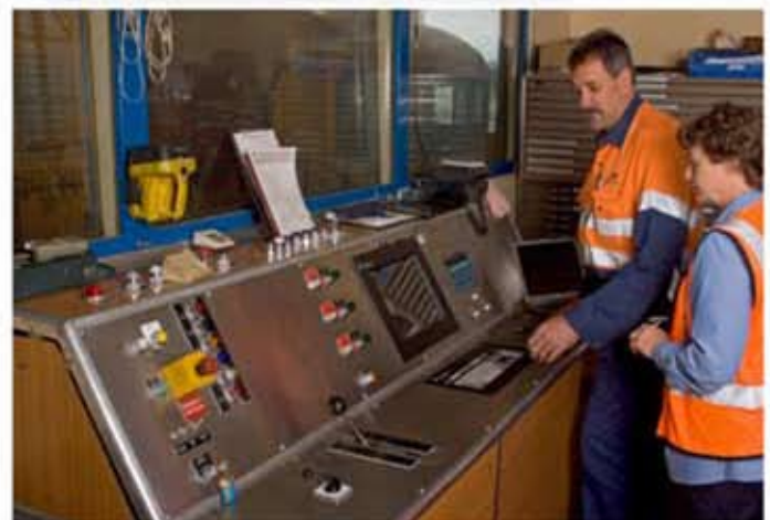
Load Box Control Room
